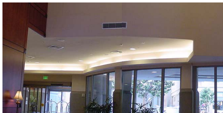
Figure 2. Thermogram/photo pair showing moisture detected on the ceiling of a hotel lobby.
